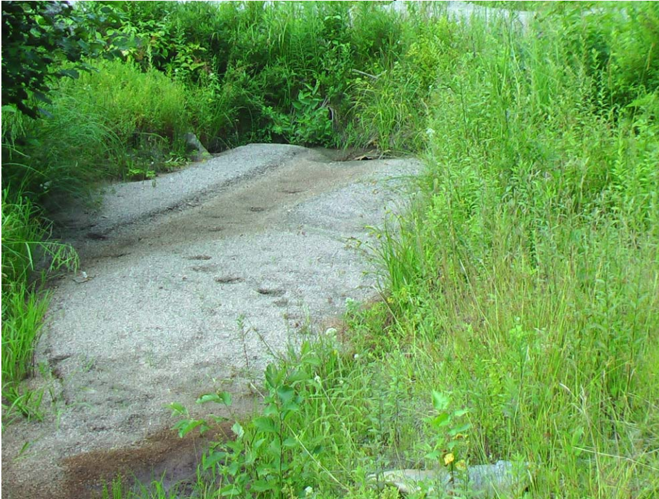
Photo 5 Stream sedimentation at culvert, July 15, 2006
